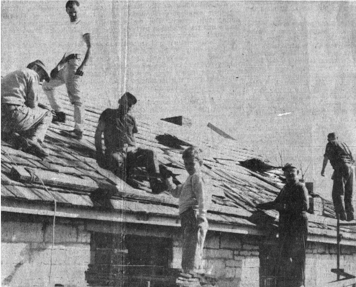
Above photo shows work bee of Muzzle Loaders organization putting new roof on the blacksmith shop which is being renovated at Fort Klock.
